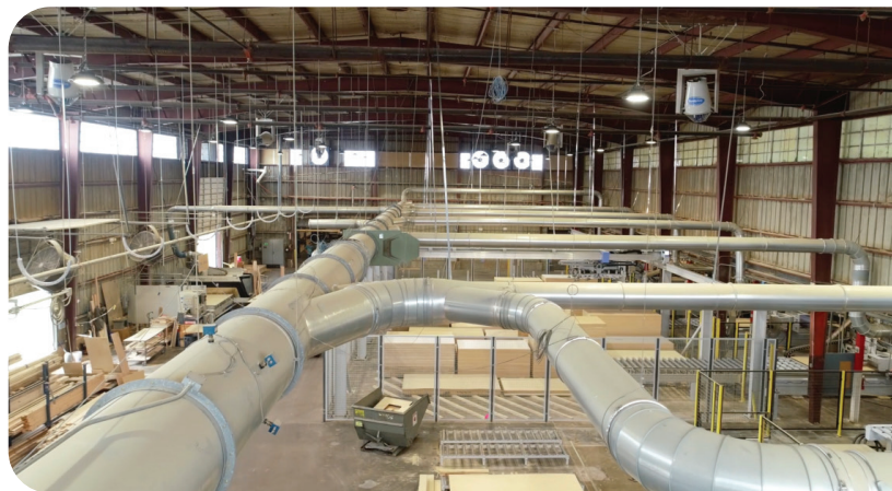
After installation and use of a SonicAire dust control system to clear away combustible dust.
